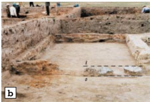
Figure 7. (a) Tilt of foundation stones (dip angle is 54^{\circ} – 75^{\circ} ) in NE direction in room No. 4; (b) uplifted modern position of stone surfaces (dashed line 1), as compared with their original position (dashed line 0).
