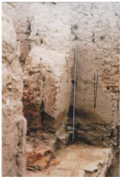
Figure 12. A SW-tilting column support of the entrance into the central chamber of the Buddhist temple.
