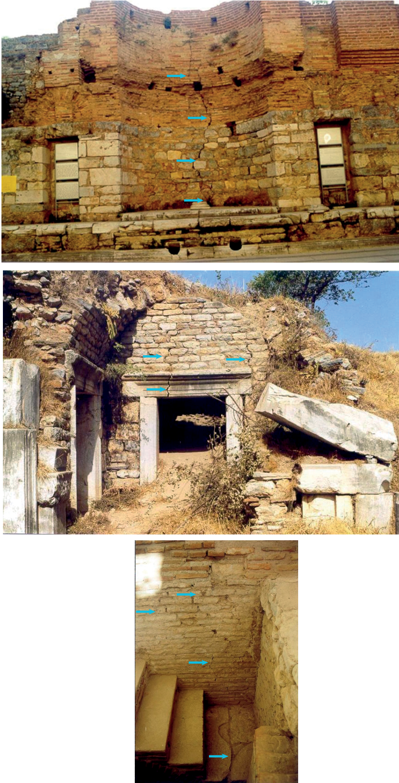
Figure 9. Possible earthquake damages (blue arrows) in the ancient city of Efes. a) western wall of the Celsus Library, b) wall of one of hillside houses, c) northern entrance of the Domitian Temple (Altunel et al., 2001).
