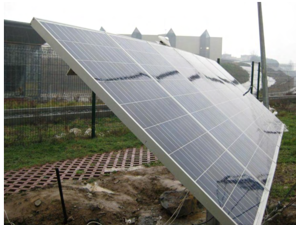
Figure 1. The installed PV system.
