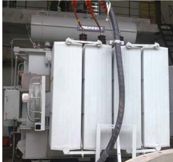
Figure 9. Picture of the filtering rectifier transformer.
