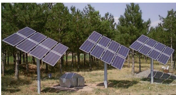
Figure 2. Overview of solar panels.
