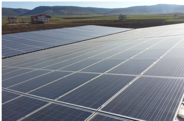
Figure 3. Photovoltaic generator installed on the roof of the textile factory.
