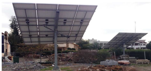
Figure 2. The 5.76 kW solar power system at CYS.
