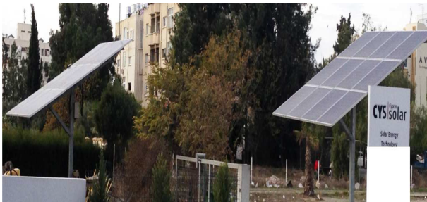
Figure 1. The 5.76 kW solar power system at CYS.
