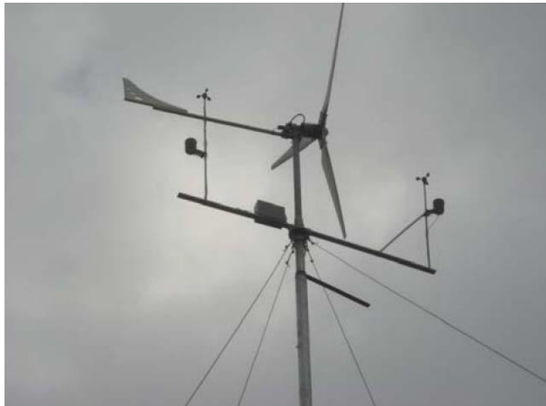
Figure 1. Illustration of the wind turbine installed.
