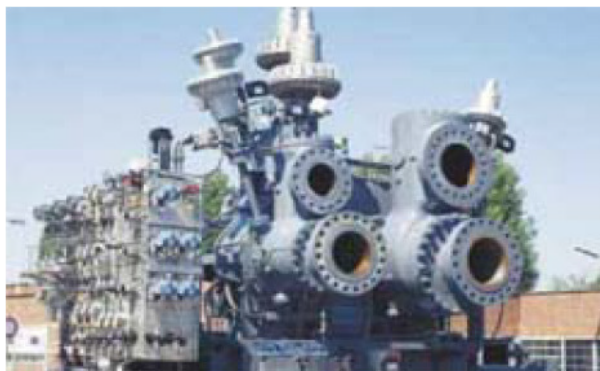
Figure 2. Turboexpander manufactured by AtlasCopco, installed in Salizone, Italy.
