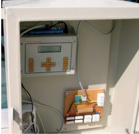
Figure 3. Current measuring circuit, data logger, and temperature sensor connections.
