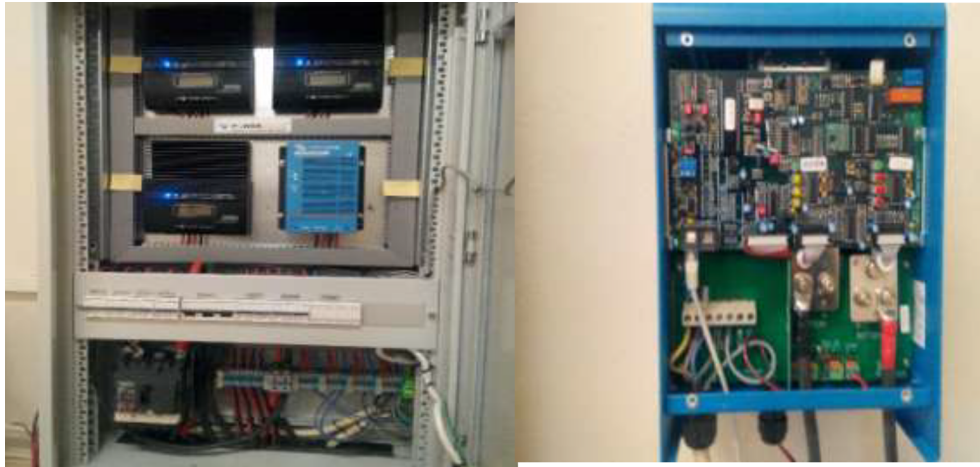
Figure 4. MPPTs and inverter.
