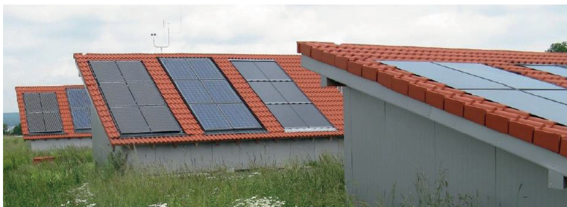
Figure 1. Three BIPV systems on rooftops with different tilt angles.
