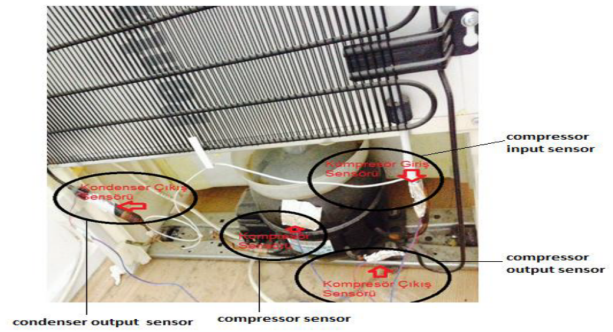
Figure 10. The rear part of the connection locations of refrigerator compressor.
