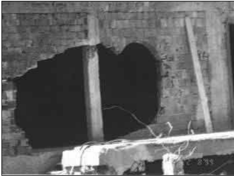
Figure 16. Out-of-plane failure of an infill wall.
