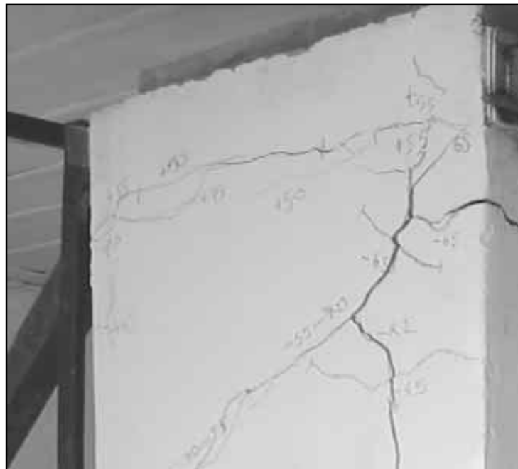
Figure 14. Close-up view of corner cracks at failure.
