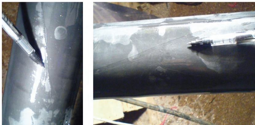
Figure 11. Effect of HF crack on impression packer plastic cover at YB station of Gotvand.
